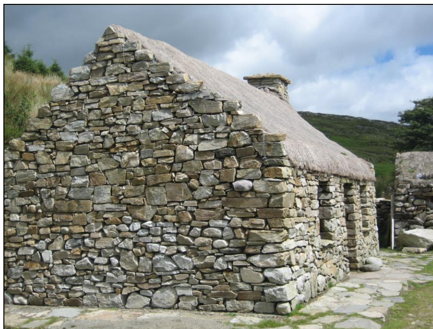
Figure 6.1. Gable view of the Dan O'Hara homestead. Photograph taken by the author.
